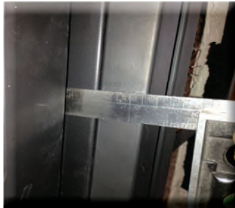
2. Measure the distance that you have for the welded tabs to go inward on the unit where the frame will be installed (in this case we have 2").
